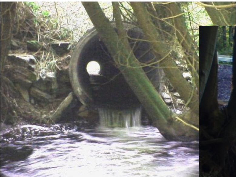
Before: old culverts obstruct fish passage
